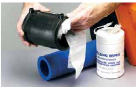
3. Use welding wipes to clean pipe and fitting surfaces. Allow cleaner to evaporate
